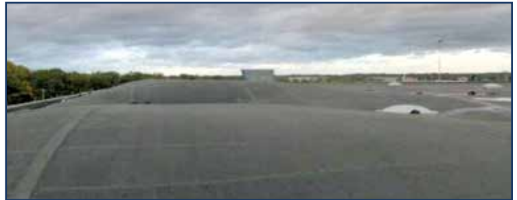
Figure 3 – Uplifted EPDM at compromised area.
