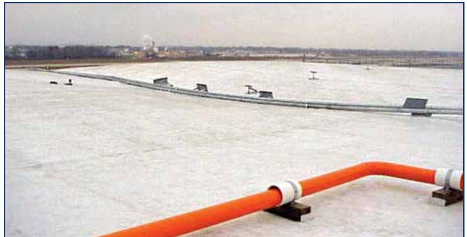
Figure 4 – Uplifted PVC roof at compromised area.
