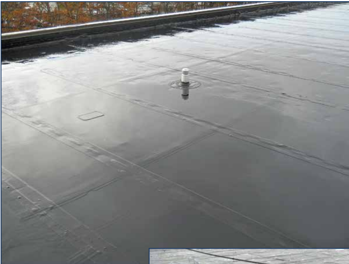
Figure 6 – Disbonded EPDM membrane area in foreground; adjacent area in background is still bonded.
