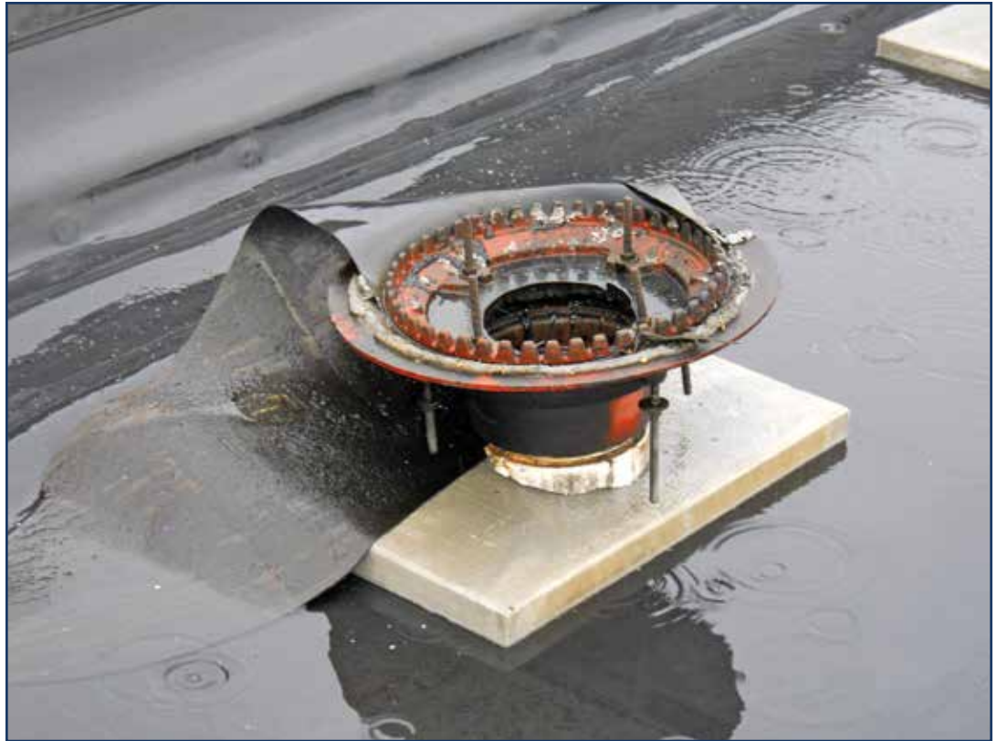
Figure 5 – Dislodged roof drain on uplifted EPDM area.
