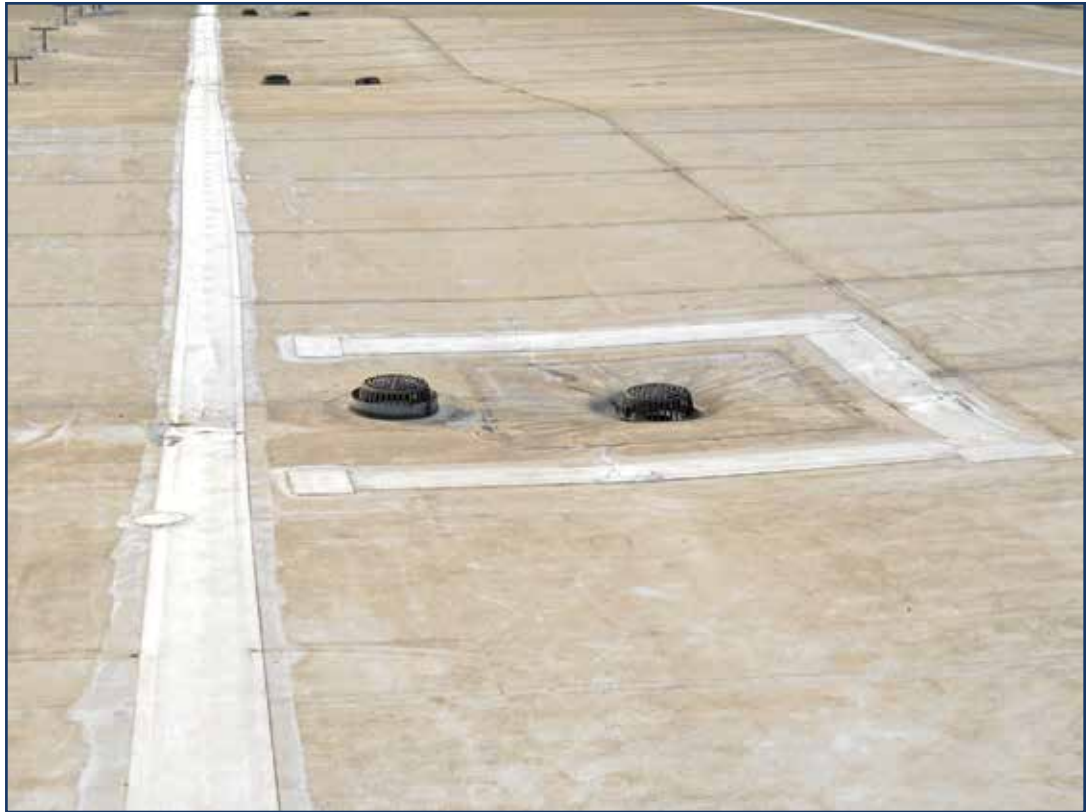
Figure 10 – Battens around roof drain on uplifted area.
