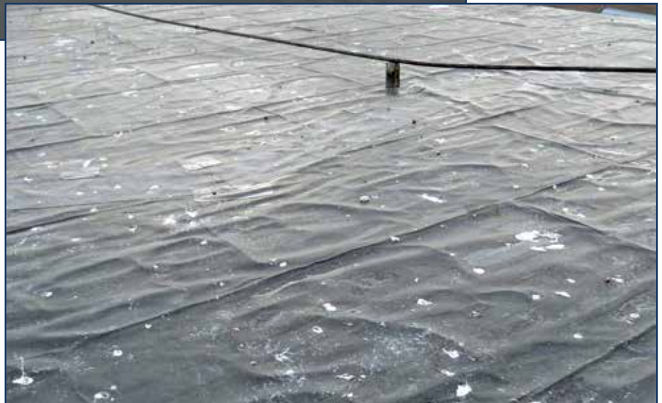
Figure 7 – Disbonded EPDM membrane with iso facer adhered to underside, pulled free of the foam core.
