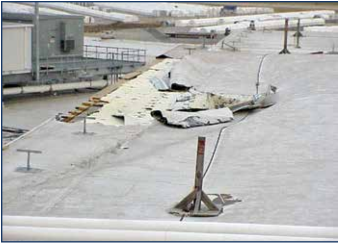
Figure 2 – Uplift damage to adhered PVC roof assembly.
