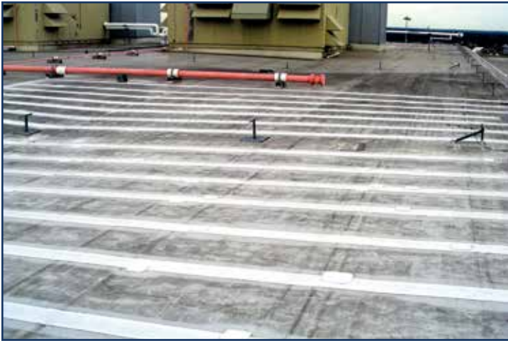
Figure 9 – Tightly clustered batten securement of an uplifted, fiberglass-reinforced PVC membrane area.
